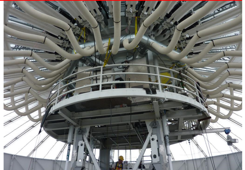
BC Place Stadion, Vancouver, Canada, air supply system made by elnic GmbH
